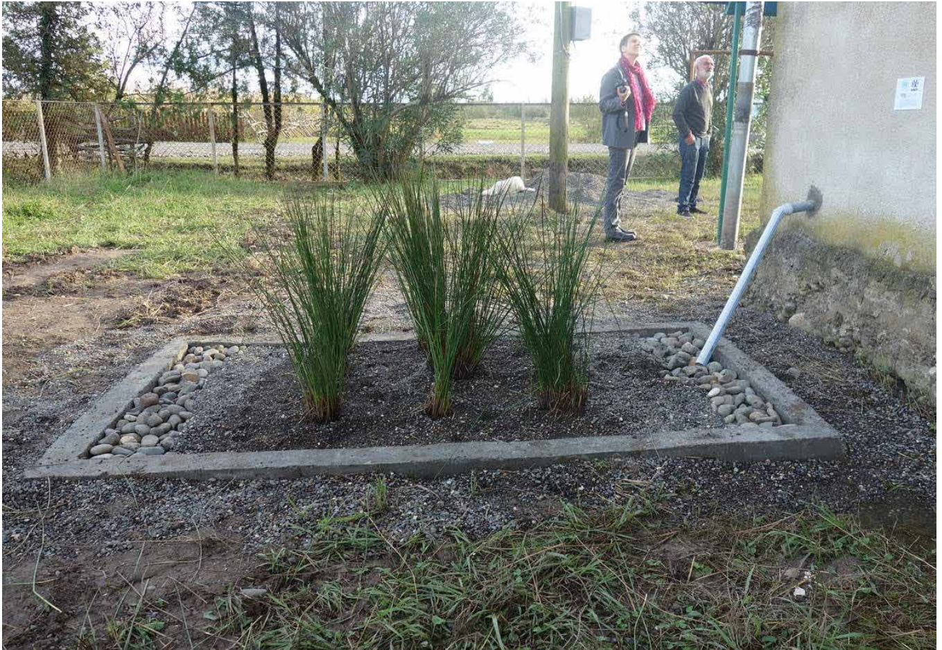
Grey water filter in rural Georgia. Source: WECF 2016.
